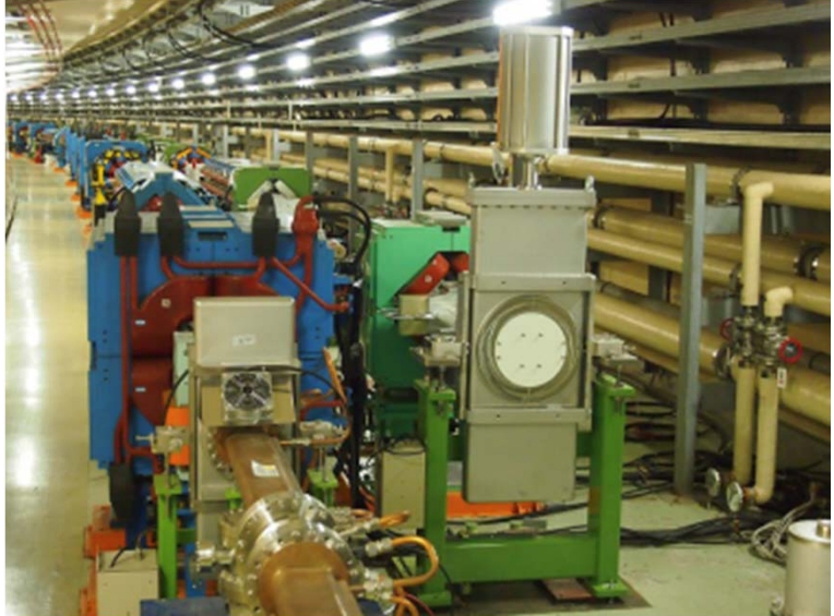
LER Gate valve in West tunnel
